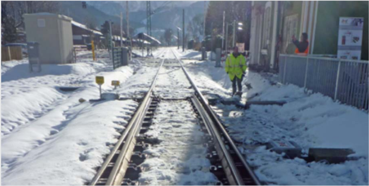
GEOKOAX probes keep railway points free of ice and snow - with zero emissions. (Photo: TripleS GmbH)
